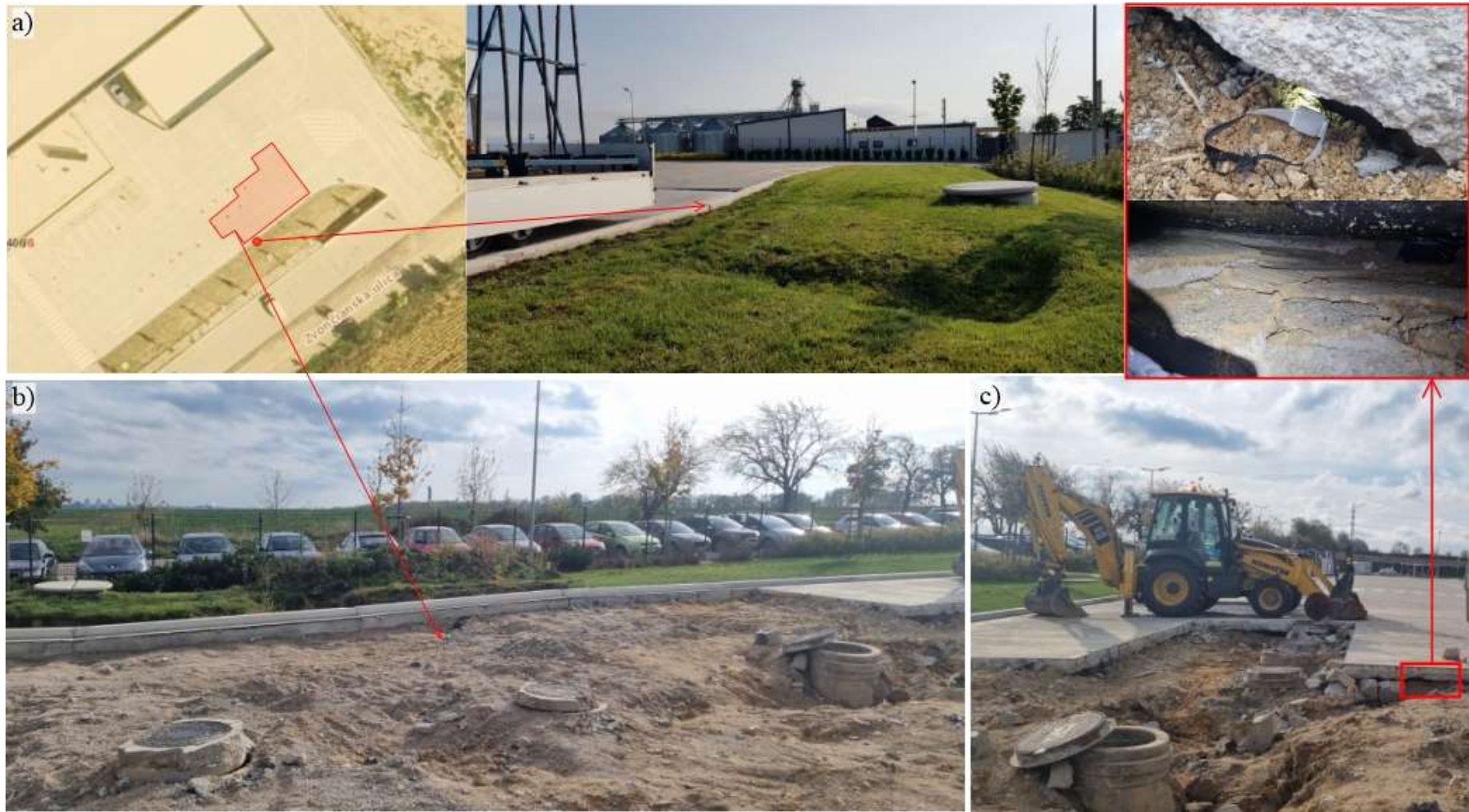
Fig. 2 Faults and voids in the front part of the area in Šelpice with their marked location (localization basis: zbgis, ÚGKK SR, Bratislava): a) curb and drainage channel collapse, b) voids between the concrete cover and the bed layer under the removed concrete slabs in the vicinity of retention tanks, c) continuation of the failure under the uncovered parts of the parking area with a detail of the cavity under the concrete slab
