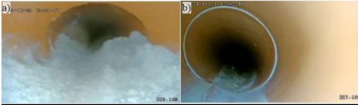
Fig. 10 Video inspection records of pipes connecting drainage elements in the area in Šelpice; a) deformations of the cross-section and deposits, b) rupture of the pipe in the longitudinal direction
