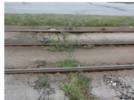
Fig. 15 Failure of the track bed
