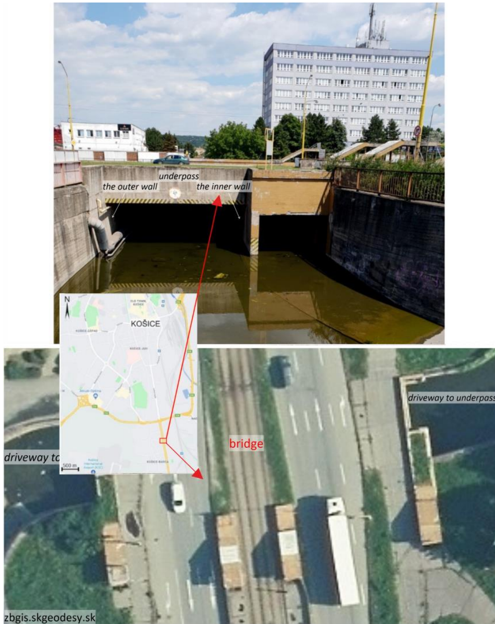
Fig. 1 The diagnosed object - a bridge with underpass to the ZŤS (VSS) in Košice
